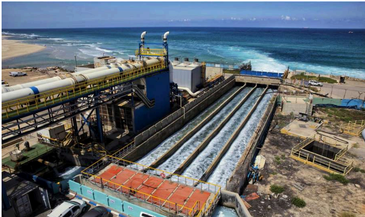
Figure 4 – Near Shore Discharge of Hadera Desalination Plant Source: IDE
