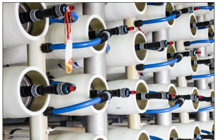
Pollutants can be removed by membrane systems including reverse osmosis.
