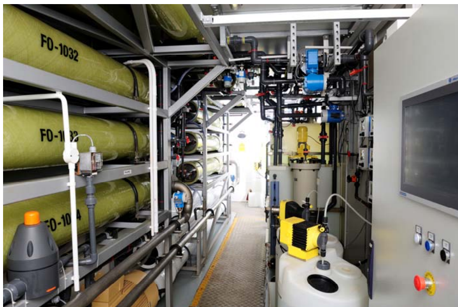
Figure 14: FO/RO desalination plant (100 m 3 /day) at Al Khaluf, Oman. Taken from [21].
